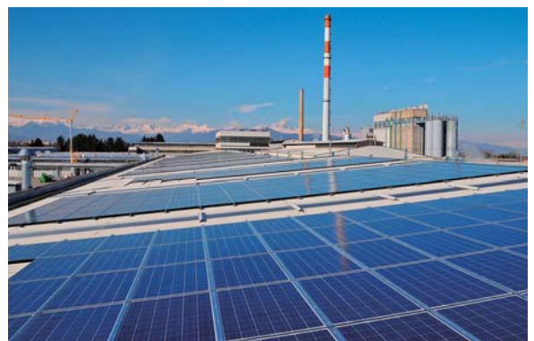
Photovoltaic panels on the roof of the Cuneo plant
