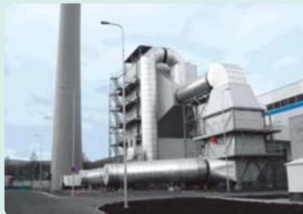
Air pollution prevention equipment installed at the Retenice Plant in the Czech Republic
