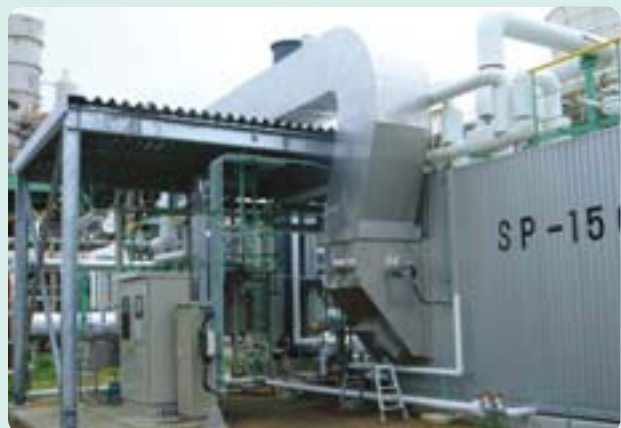
Hydrogen boiler contributing to substantial CO 2 emission reductions
