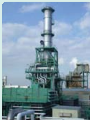
Gas turbine power generator newly introduced to the Chiba Plant
