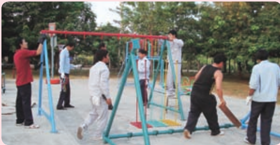
Employees engaged in assembly and construction work on a weekend tour to the site
