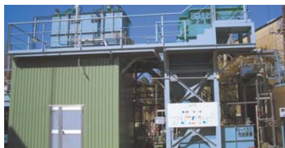
Groundwater pumping and decontamination facility (Seimi Chemical)
