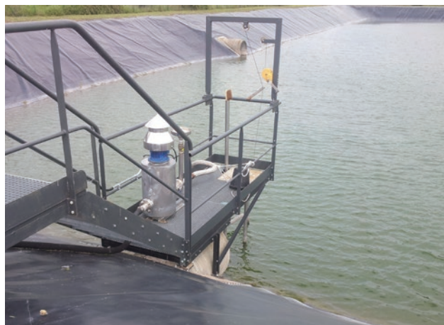
Storm water recovery system in Seingbouse, France.
