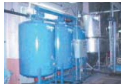
Sand pressure filter system for elimination of glass sludge
