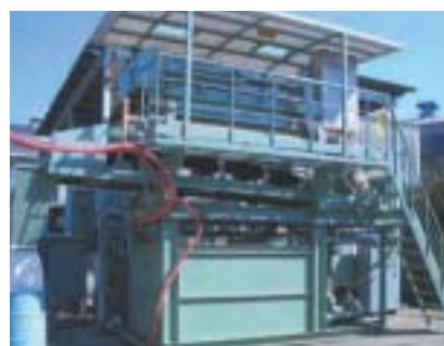
Groundwater decontamination pumping equipment installed at Chigasaki Plant site
