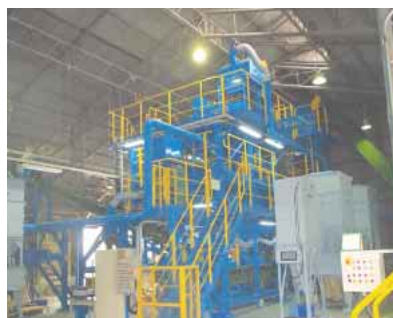
Equipment for sorting glass (after crushing)
