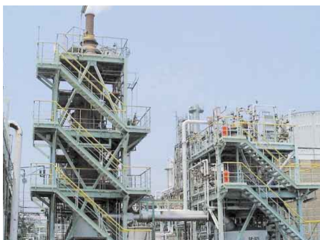
CFCs destruction plant
