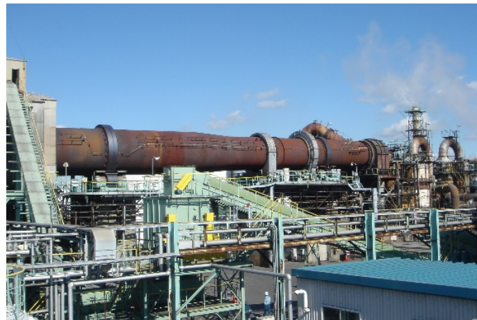
A combustion facility at JX Nippon Tomakomai Chemical
